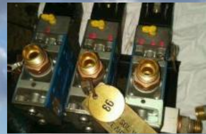
Fixed CO2 system service
