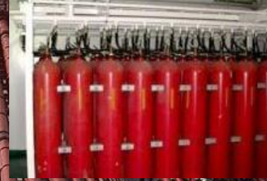
Fixed CO2 system service
