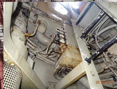
Cargo Crane hydraulic service
