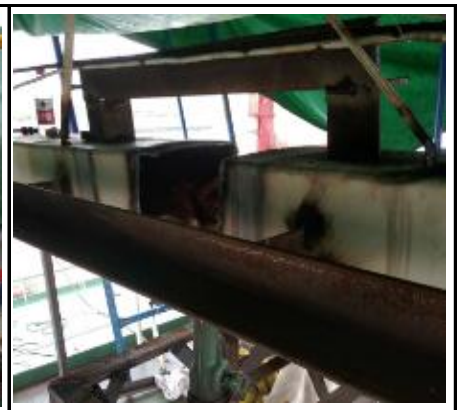
Reinforced to protect the jib from distorting
