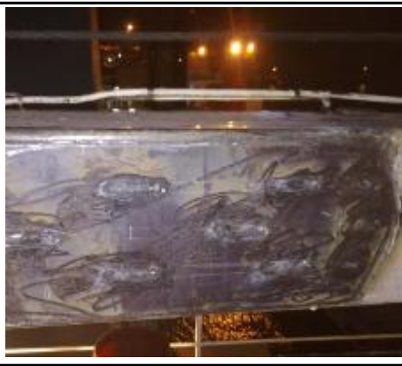
Fitted up ,welded and ground the reinforcement (double plate locating on both sides)
